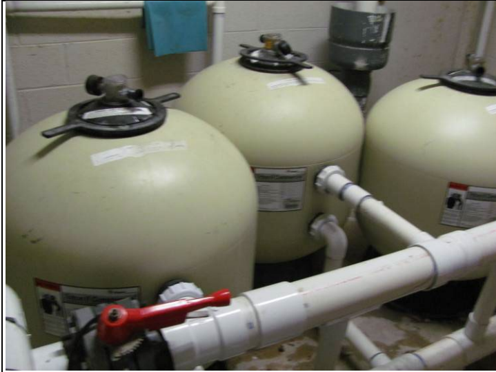
Photo #4: Main pool filter
