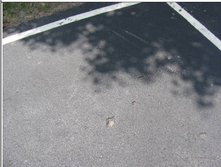
Photo #9: Basketball court damage
