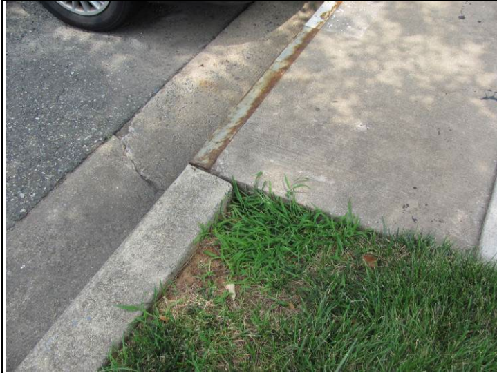
Photo #22: Sink hole by drain curb
