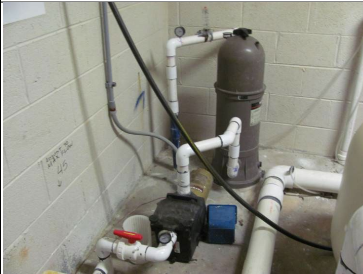
Photo #2: Pool filter system for wading pool
