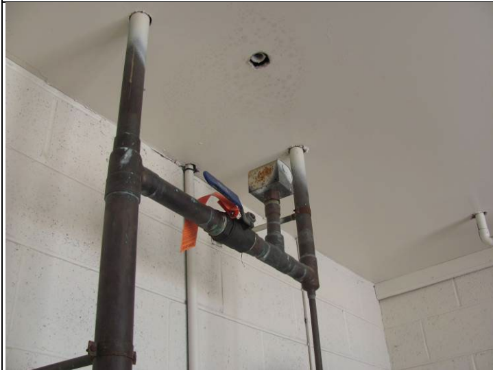
Photo #5: Pool office with sprinkler head removed
