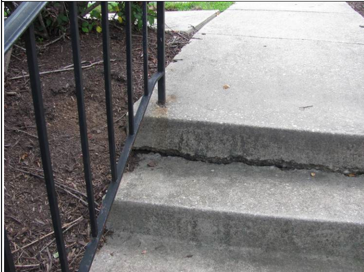
Photo #23: Stair system settling
