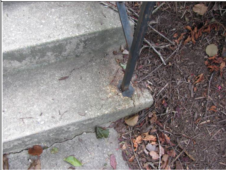
Photo #24: Stair post set depressed
