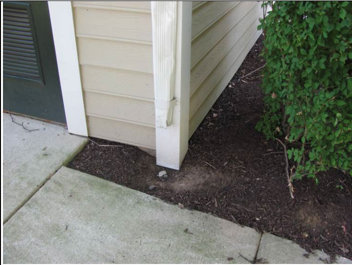
Photo #1: Downspout boot missing
