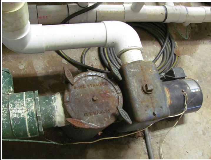
Photo #3: Main pool pump
