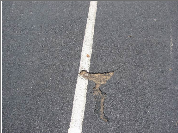
Photo #8: Basketball court damage
