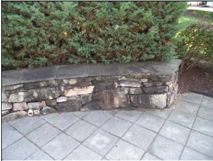
Photo #29: Consideration should be given to washing the retaining wall.
