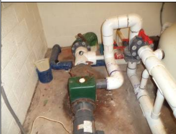
Photo #3: Main pool pump
