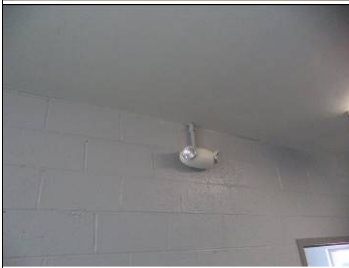
Photo #9: Pool house emergency lighting
