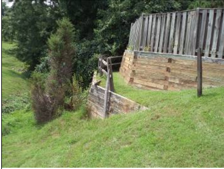
Photo #55: The split rail fence by the drainage field is damaged, and deteriorated areas require some repair.
