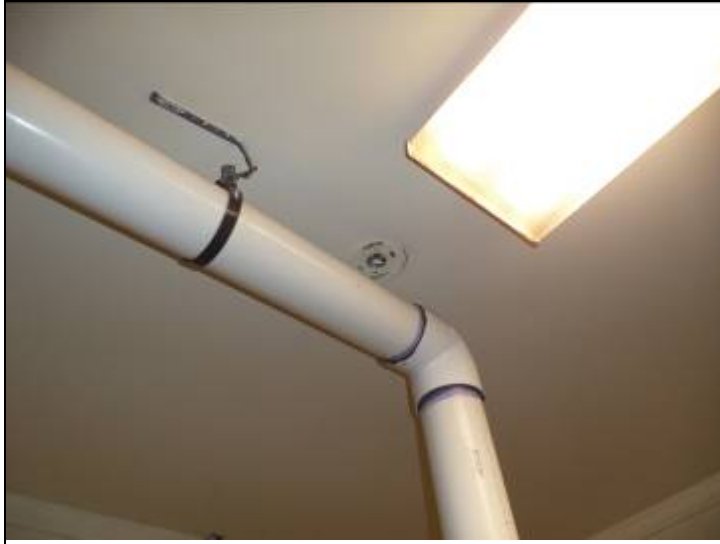
Photo #7: The smoke detector in the pump room has been removed. We recommend that this be reinstalled.
