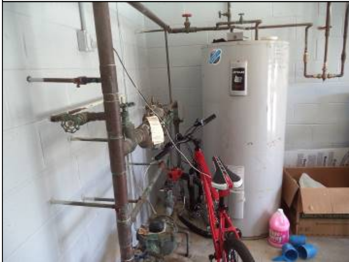
Photo #11: Last domestic water heater
