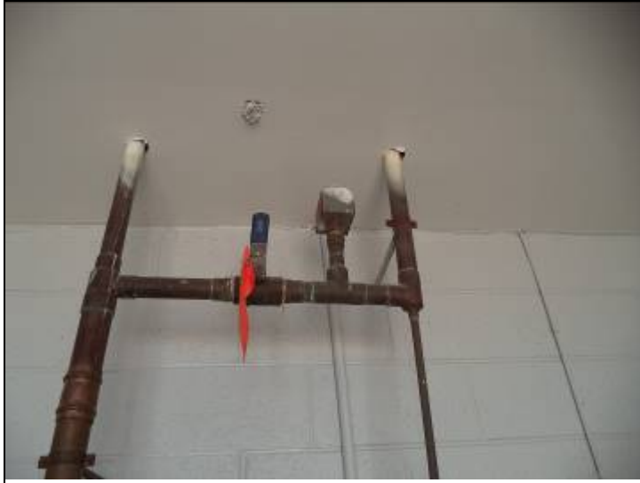
Photo #13: The sprinkler system for the pool house has been isolated, and the heads have been removed.
