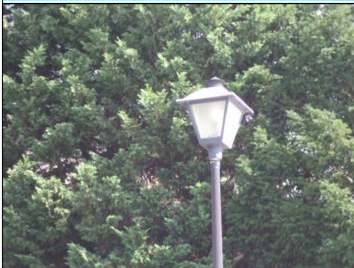
Photo #18: The light fixtures are still operational. However, the finish of the fixture heads are worn and should be refinished.
