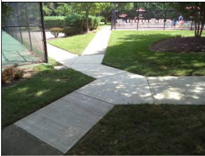
Photo #27: Management has replaced some of the damaged concrete on the property.
