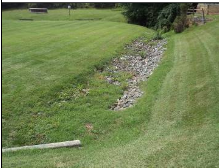
Photo #54: The riprap is starting to have some overgrowth, which will reduce the efficiency of the riprap. The riprap does require some attention.
