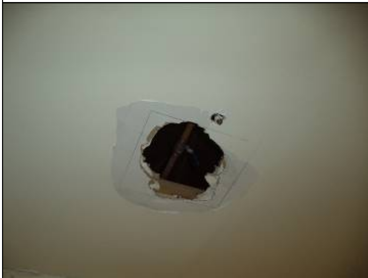
Photo #8: There is an open ceiling in the pool pump room where a domestic isolation valve has been installed. A proper access panel should be installed this location.
