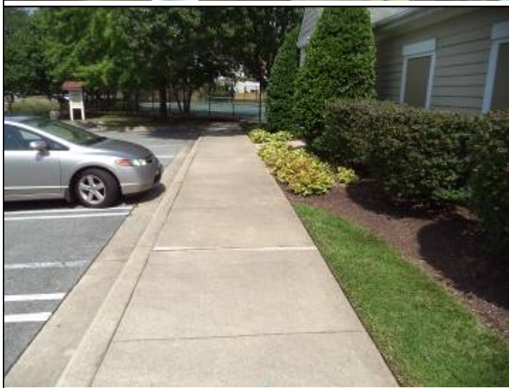
Photo #24: The management committee has had the concrete in some areas ground to prevent trip hazards.
