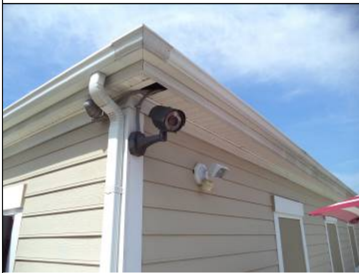
Photo #21: Pool house camera
