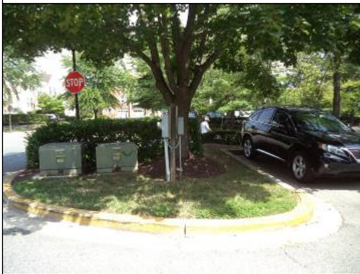
Photo #60: Electrical service for the front entrance sign lighting.
