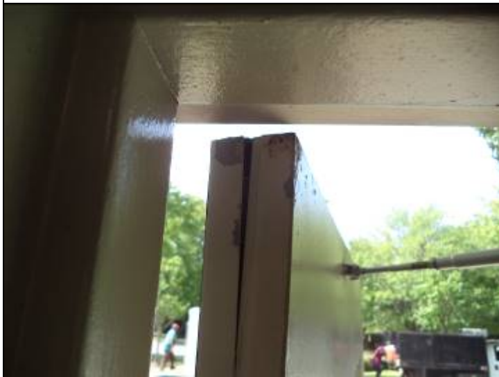
Photo #23: The entry door at the pool house is damaged where the metal is splitting. This should be sealed to retard deterioration.
