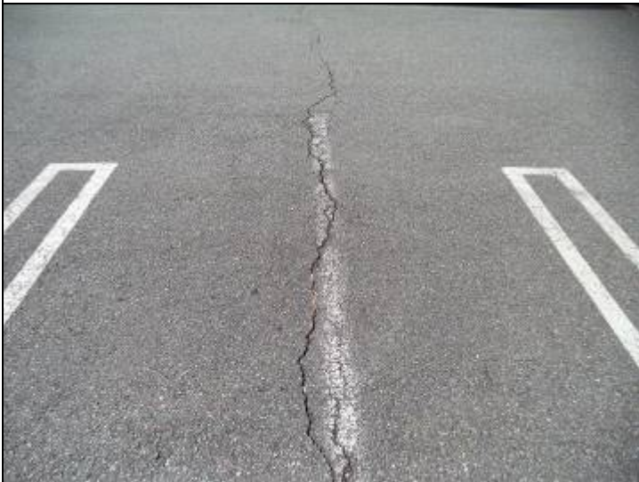
Photo #2: There is a crack in the asphalt surface at the pool area, which we recommend be sealed with a hot liquid asphalt material.
