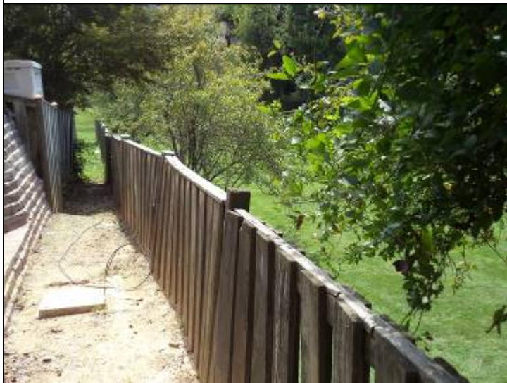
Photo #53: The fence along this walk has deteriorated and requires repair.
