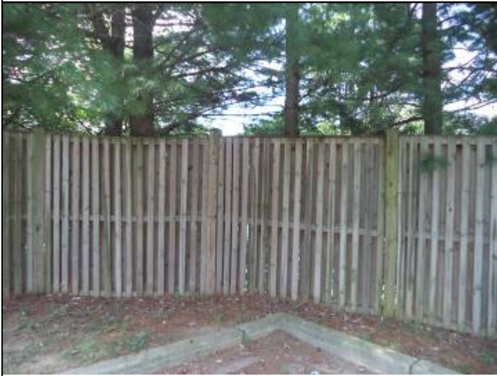
Photo #41: The sound wall fence has had repairs made in a few areas.
