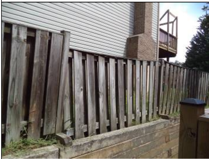
Photo #45: Some of the fences on top of the walls and some of the walls are deteriorated. These require repairs and restoration.
