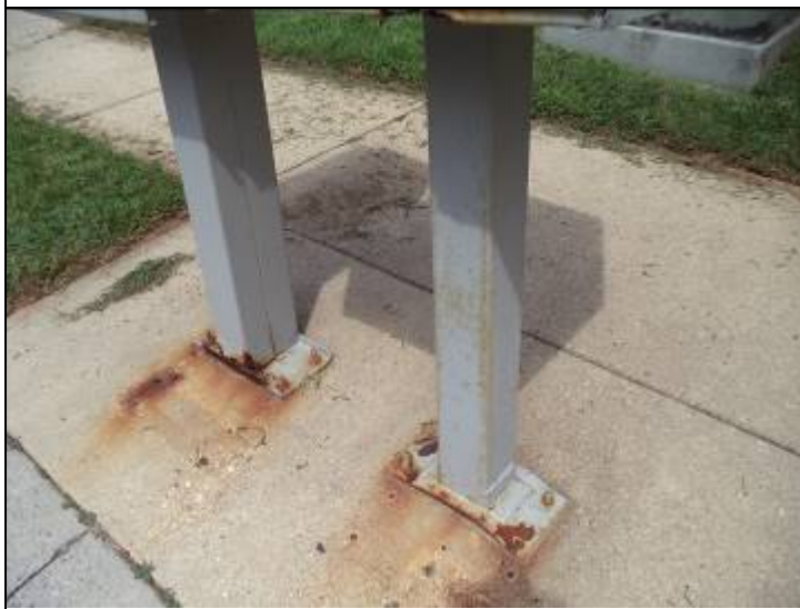
Photo #48: Some of the original mailboxes have some deterioration of the base metal. We recommend these be addressed to prevent full deterioration.
