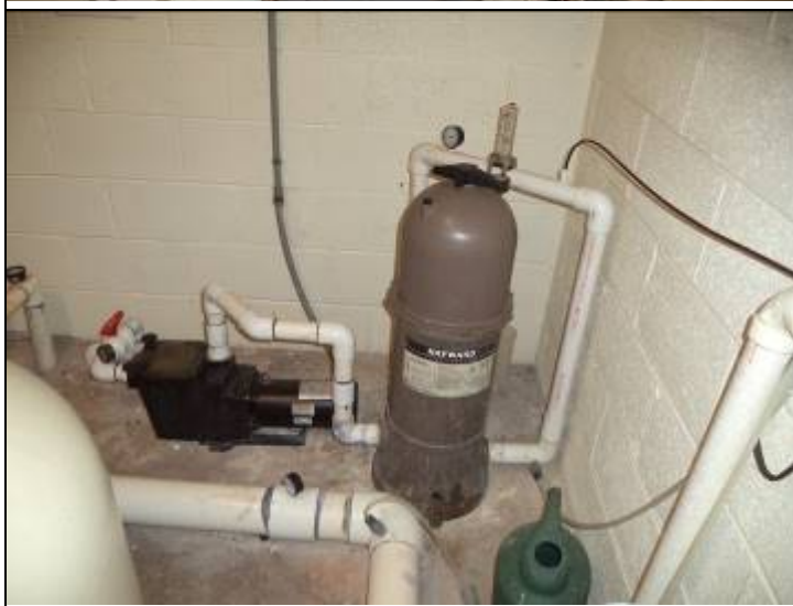
Photo #6: Wading pool filter and pump
