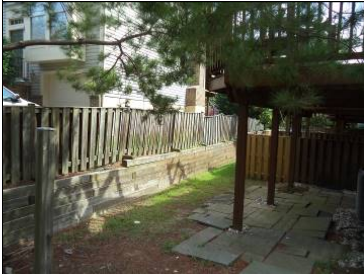
Photo #44: Some of the fences on top of the walls and some of the walls are deteriorated. These require repairs and restoration.
