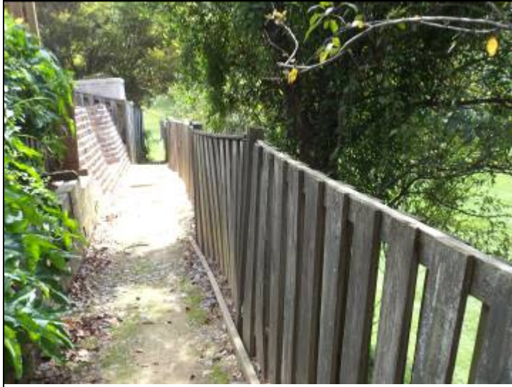
Photo #52: The fence along this walk has deteriorated and requires repair.
