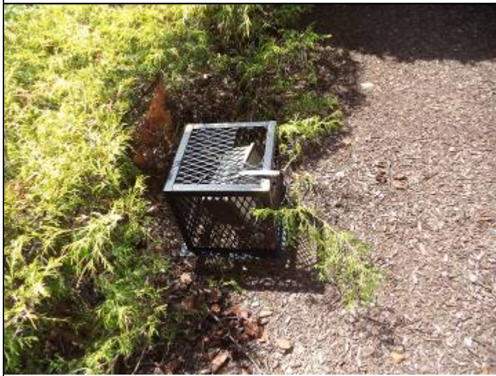
Photo #62: Entrance monument lights
