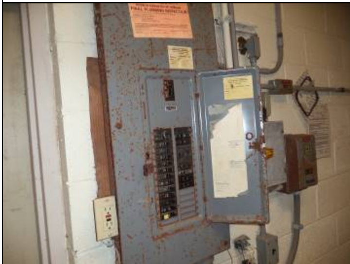
Photo #5: The electrical circuit panel box is oxidizing, which is not unusual in the high humidity pump rooms for pools. This should be monitored to ensure that a safe condition is maintained.
