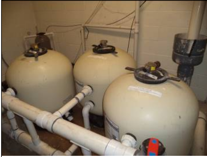
Photo #4: Main pool filters
