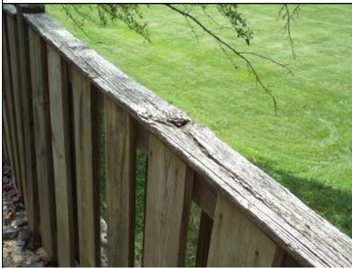
Photo #51: The fence along this will walk is deteriorated and requires repair.
